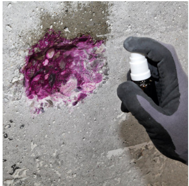
Here, the concrete provides adequate protection. The violet color indicates that the concrete is sufficiently alkaline.
