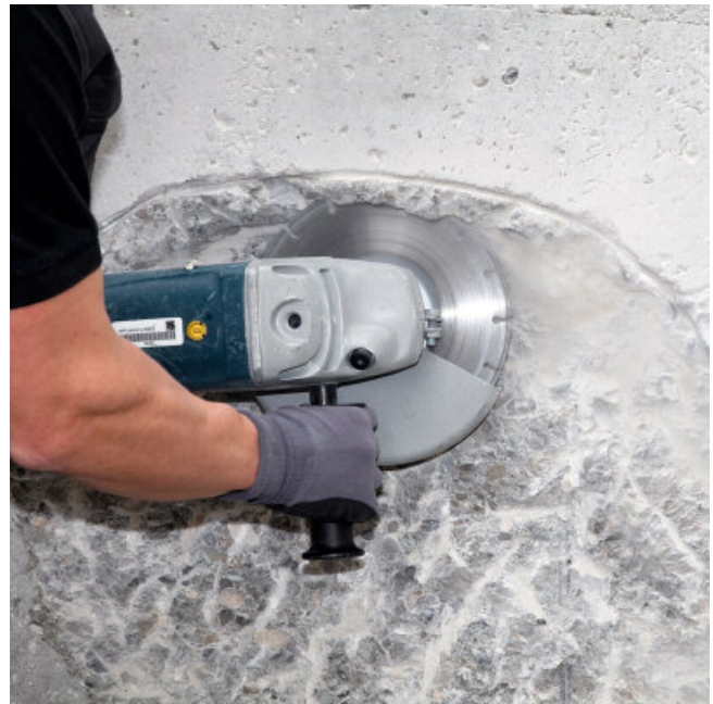
Clean cutting of the edges ensures a tidy transition and optimum adhesion of the repair mortar.
