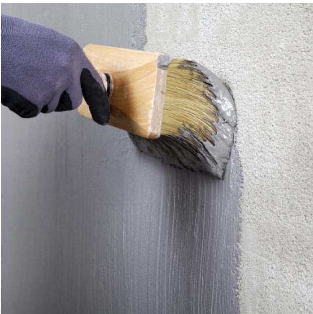
Exterior waterproofing of a foundation wall using PCI Barraseal® Turbo, which can be applied using a brush or trowel.
