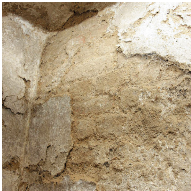
Cellar with moisture and salt damage prior to refurbishment
