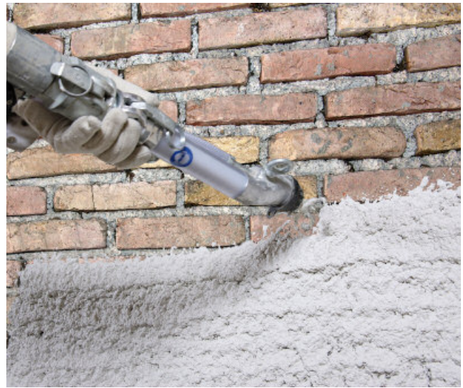
Application of one layer of PCI Saniment® 2 in 1 to the inside of a basement wall
