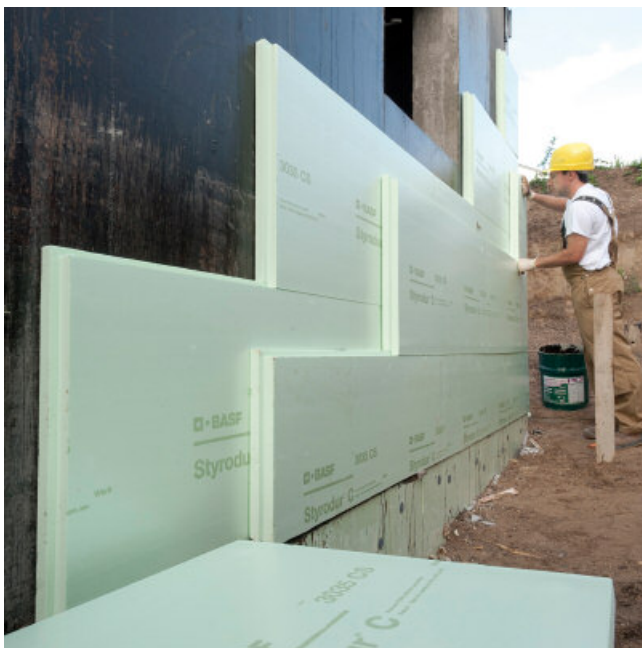
Bonding of insulating boards with PCI Pecimor® 2K or the insulating board adhesive PCI Pecimor® DK
